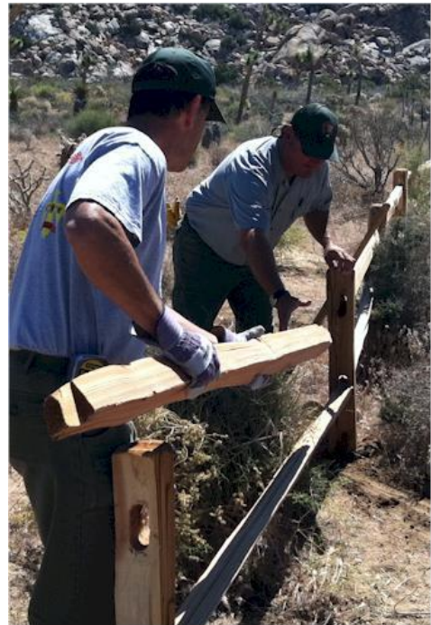
The OA hard at work replacing a split-rail fence in Joshua Tree. (Photo: M. Hare)
