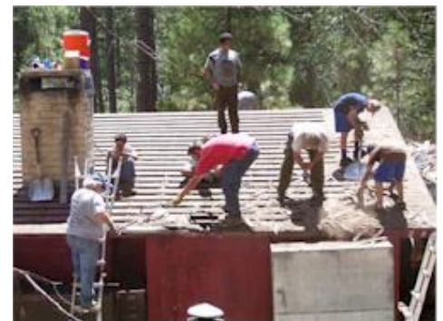
Members of Cahuilla Lodge work on a reroofing project on Boyce Lodge at Camp Emerson (Photo: S. McLeod)
